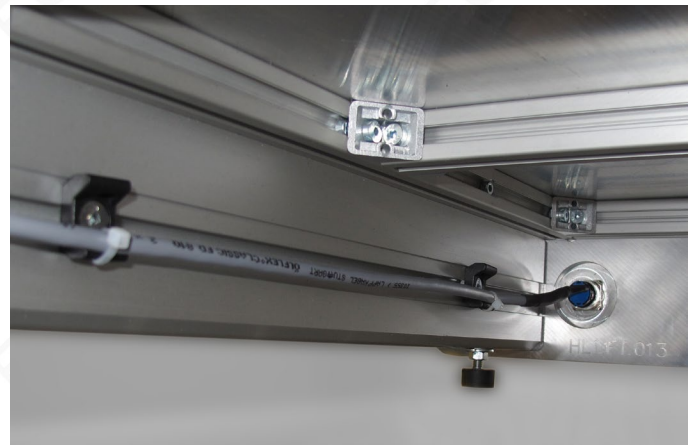
Fig. 7: Control line to the emergency stop switch
