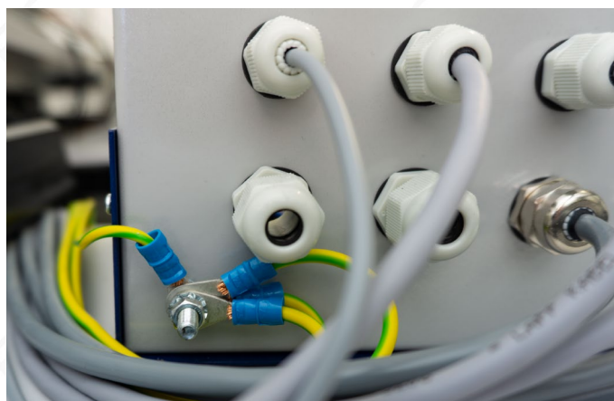
Fig. 2: Central ground point on the housing of the controller
