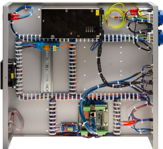
Fig. 21: Power supply cabling and axis connections
