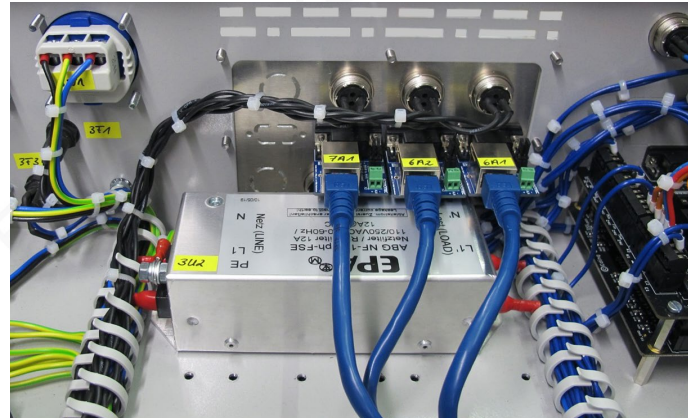
Fig. 2: Line filter in front of the output panel
