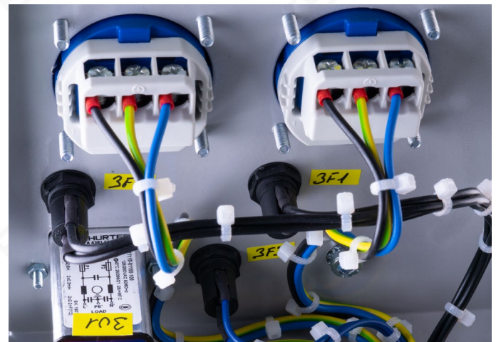
Fig. 14: The sockets for cooling and milling spindle
